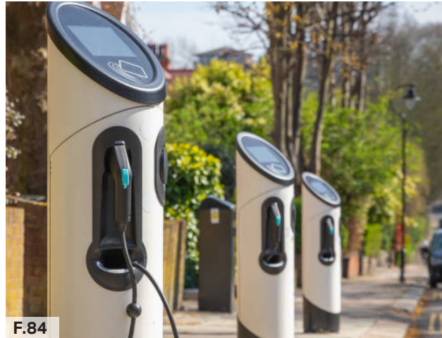
Figure 84: Examples of on-street car charging points.
