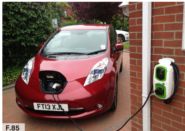
Figure 85: Examples of off-street mounted car charging points.
