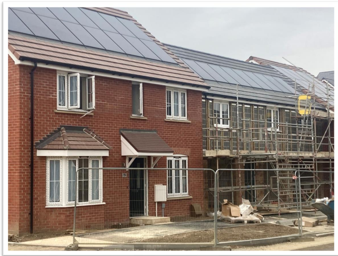
New build with roof solar panels
