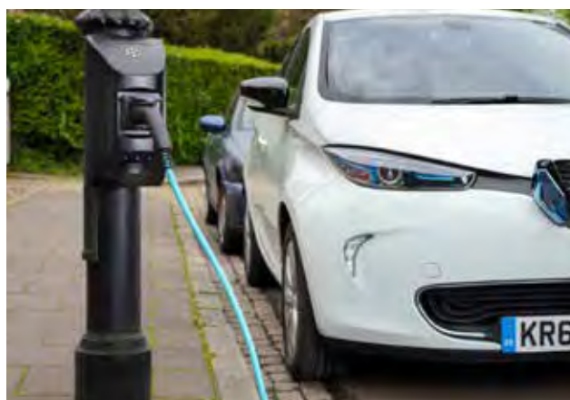
Figure 59: Example of on-street electric vehicle charging points.
