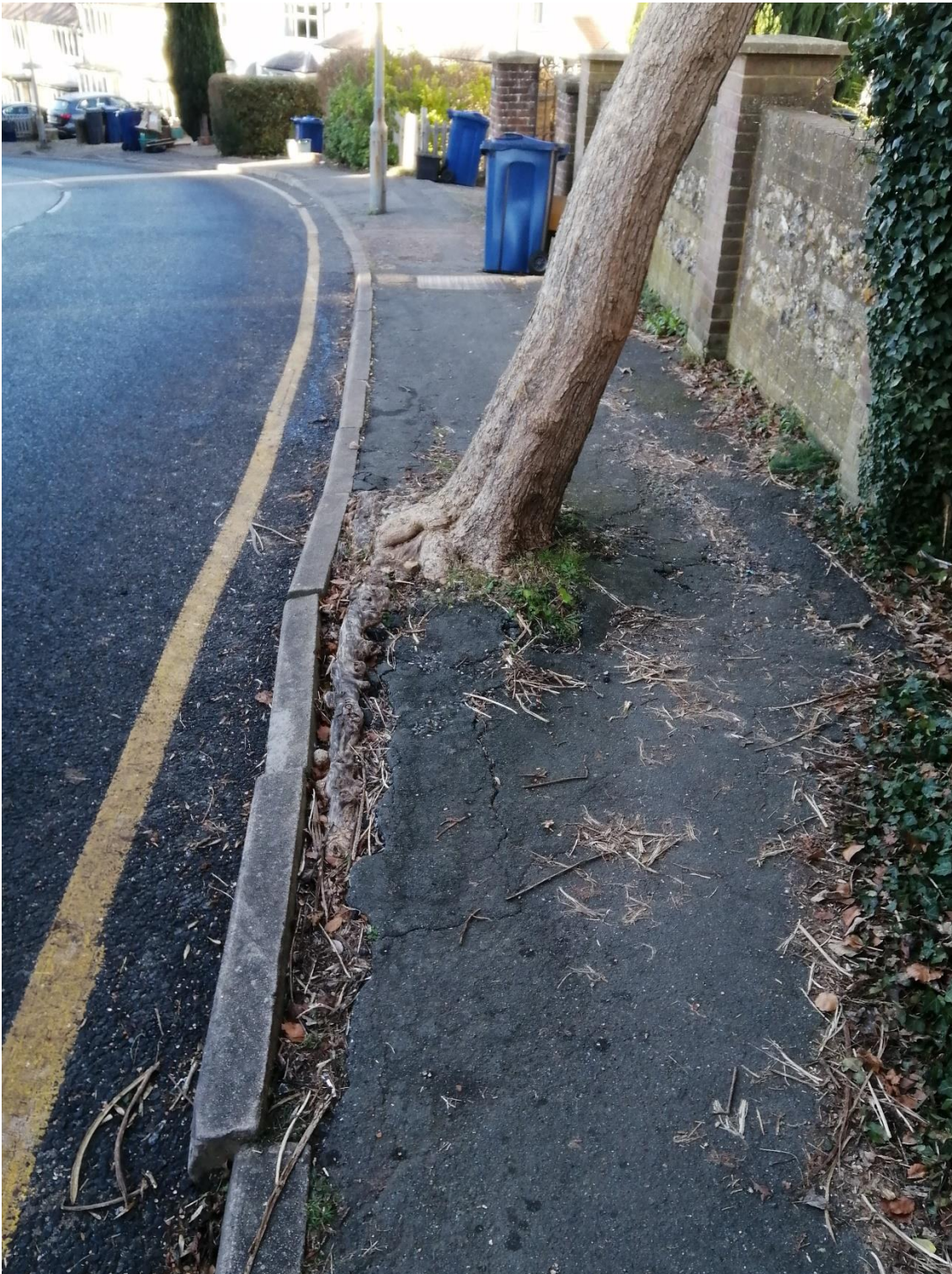
Figure 24: showing the leaning stem of the catalpa T009, with buttress roots extending along the kerb, causing displacement of kerbstones. Pedestrians with wider buggies must detour into the road to pass the tree.
