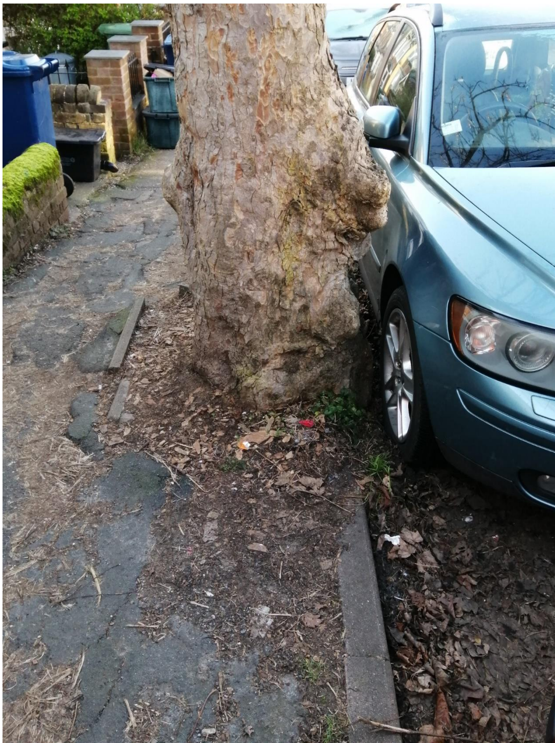
Figure 23: showing limited space for pedestrian passage, uneven surfacing and displaced edging units at the base of the sycamore T002.
